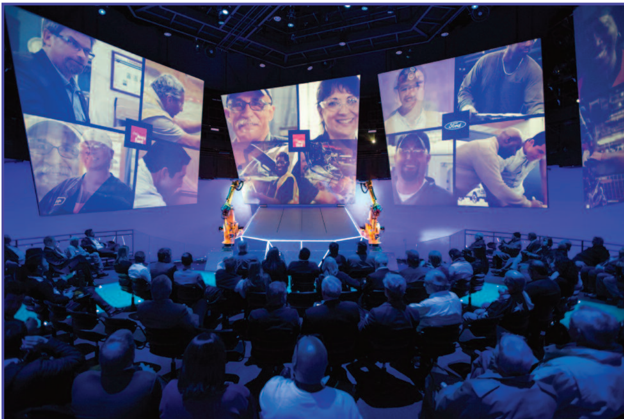
Existing projectors and screens were reconfigured and updated with new equipment and control systems.
