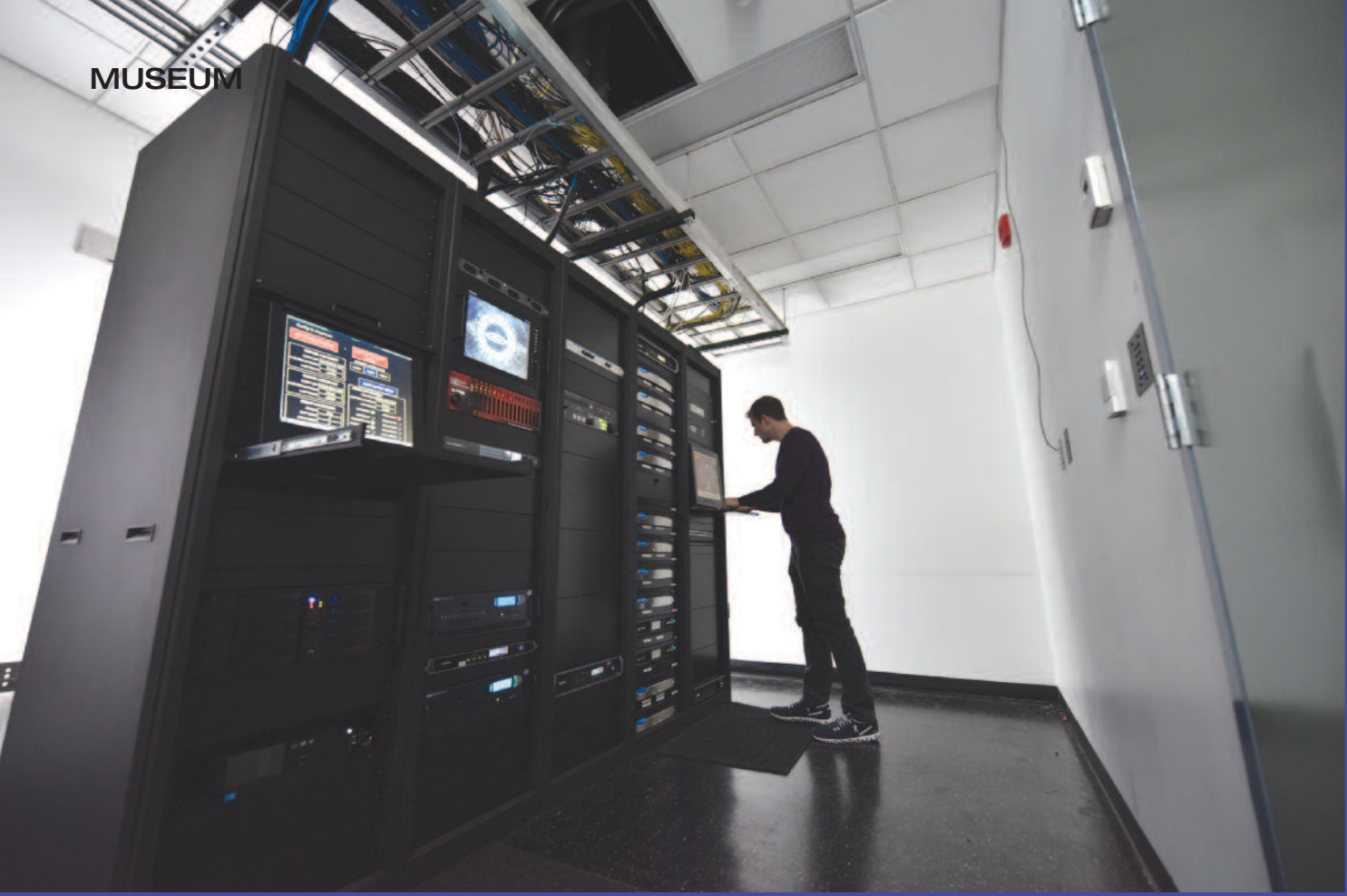
The main show control panel for the facility lives in the equipment room upstairs.
